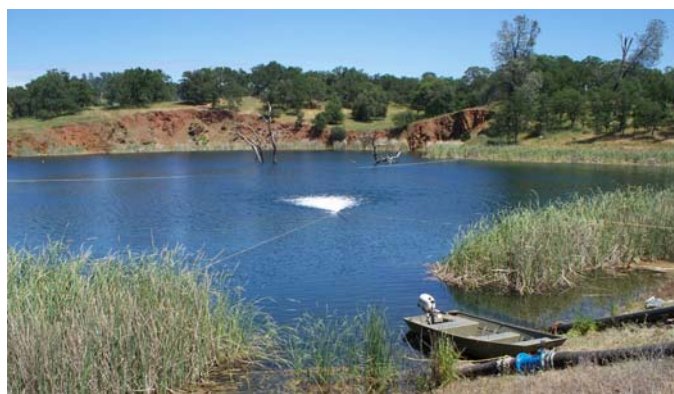
A simple pump on a boat distributes an iron sulfate solution that demonstrated successful removal of arsenic from Skyrocket Lake during a pilot study.
